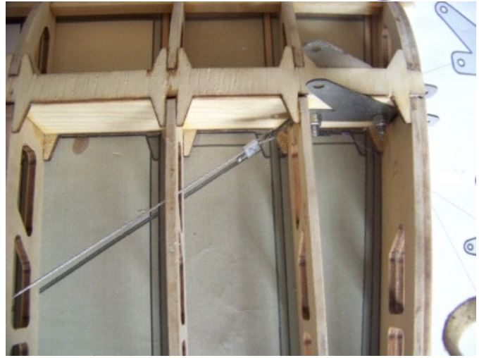
(11) Joint rib E1. And fix the wing on the installation drawing again, then pull \phi 0.8mm steel wires.
